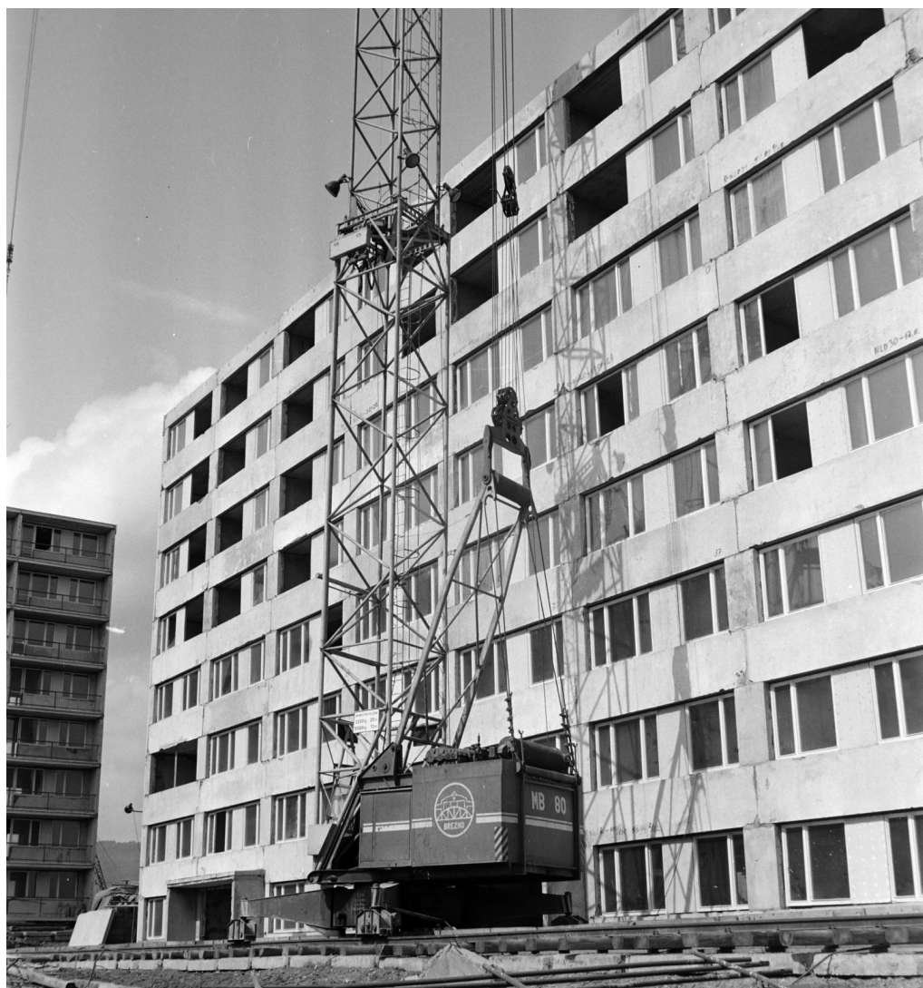
The construction of the residential area called Košice-West. On the left, it is block no. 4-14 of Trieda SNP (1964). (Fortepan/photo by Viktor Gábor)
